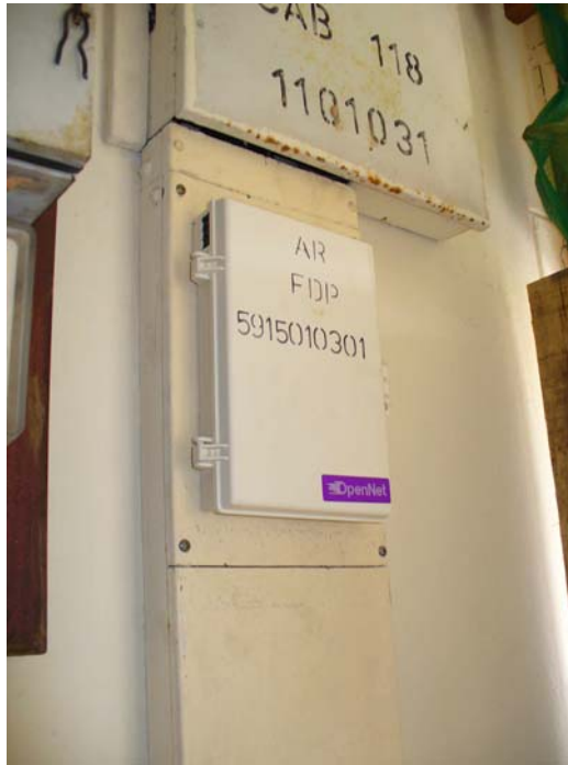
Figure 22: Photograph of a Wall-mounted Fibre Termination Box (Courtesy of OpenNet Pte Ltd)
