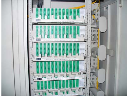
Figure 24: The Interior of a Termination Cabinet (Courtesy of OpenNet Pte Ltd)
