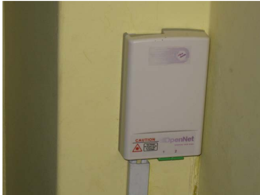
Figure 3: Wall-mounted termination box (Courtesy of OpenNet)
