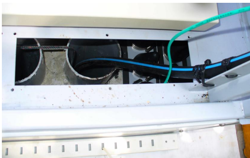
Figure 16: Fibre Cable in a Conduit (Courtesy of OpenNet Pte Ltd)
