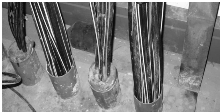
Figure 17: Underground Conduit with Cables (Courtesy of OpenNet Pte Ltd)
