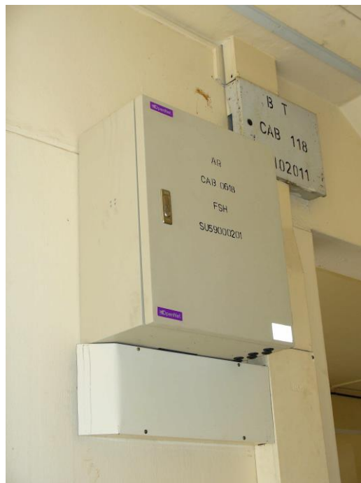
Figure 23: A Wall-mounted Fibre Distribution Box (Courtesy of OpenNet Pte Ltd)
