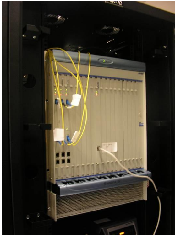
Figure 3: Optical Line Terminal (OLT) Equipment
