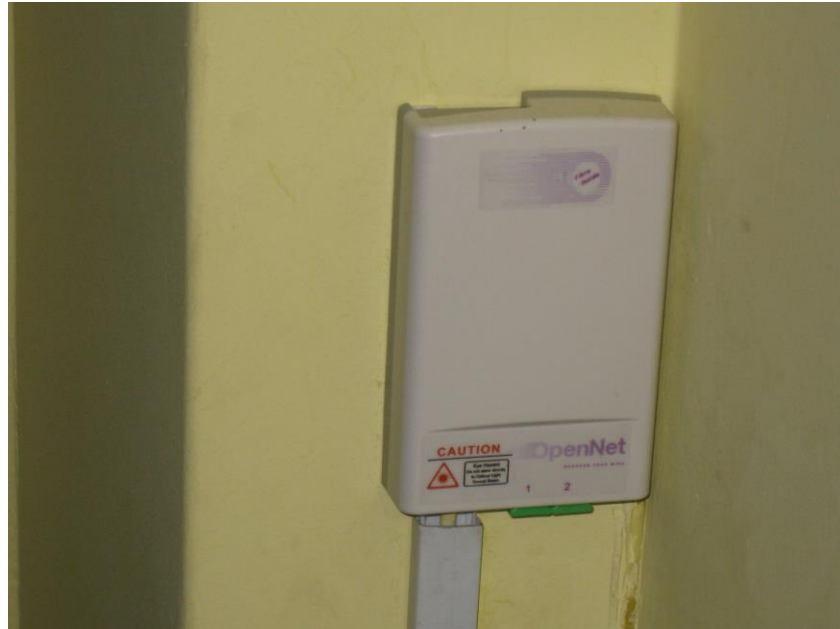
Figure 3: Wall-mounted termination box (Courtesy of OpenNet)
