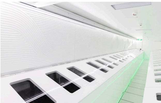
Row of immersion cooling tanks
